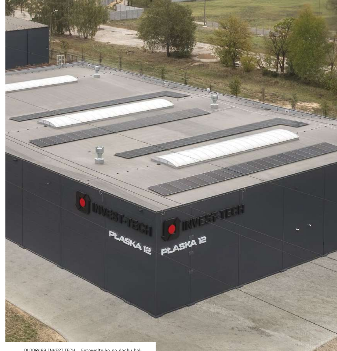
PL006488 INVEST-TECH – Fotowoltaika na dachu hali
